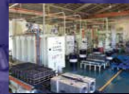
Vacuum heat treatment facility in Incubation plant
